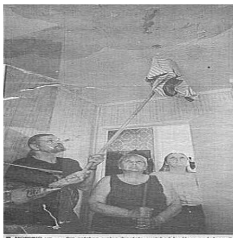
Damage caused by the water in the Rochdale home.
